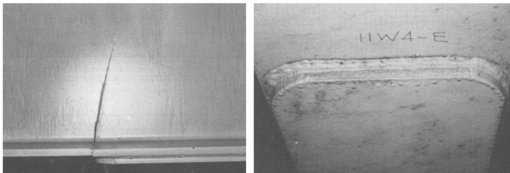
Figure 4.8: Fatigue Cracks at Cover Plate Details in the Yellow Mill Pond Bridge (Fisher, 1984).
